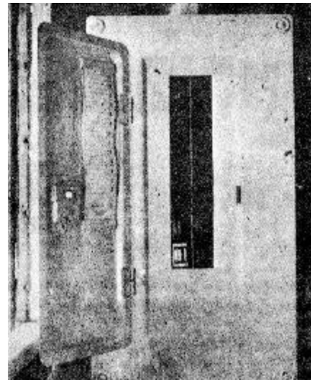
Figure 4. Electrical control panel and identification list.
